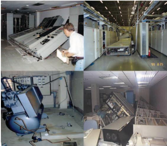
Figure 1. Damage of non-structural components. 19
